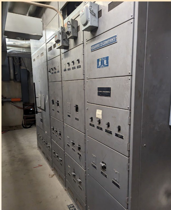
HS Electrical Panel
